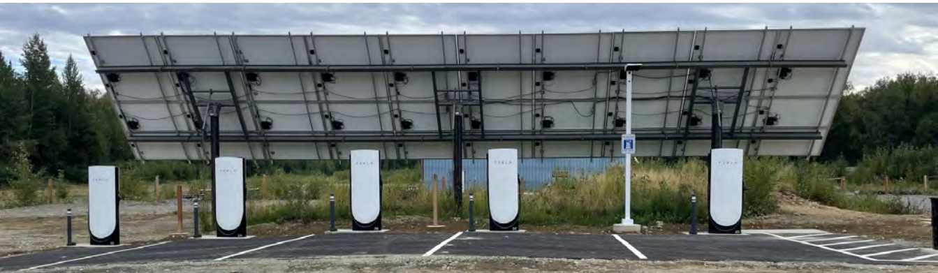
EVSE along the AFC.
